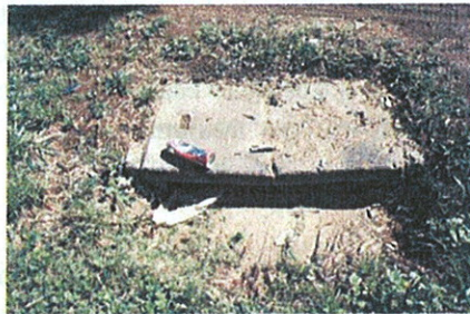
Plate 4: Typical Stormwater Pit in Nurra Reserve
